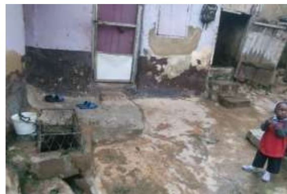
Plate 1.6: Safe distance of 2.8m between soakaway pit and well in Kawo high density Source: Author's Field survey, 2020.
